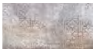
AVEYU3060820 | white rust
